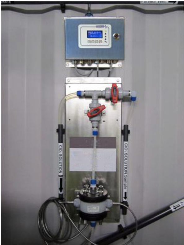
Kemtrak chlorine dioxide analyzer installation
